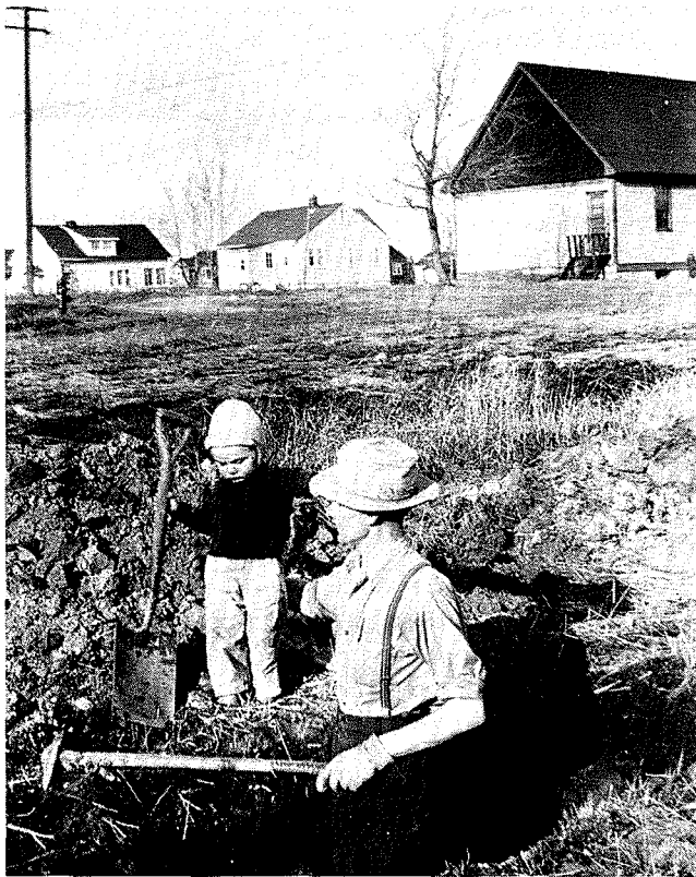
Stan Levitt and son Fred in 1944 digging a ditch for the sewer for their new house.
